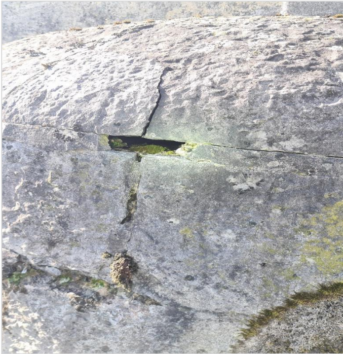
Plate 3-4: small crevice in abutment.
