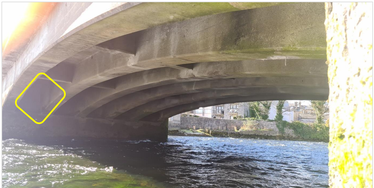
Plate 4-1: One of the 6 locations (yellow section) where concrete will be set in the outer valley. No evidence of bats was found in this outer valley of the bridge.
