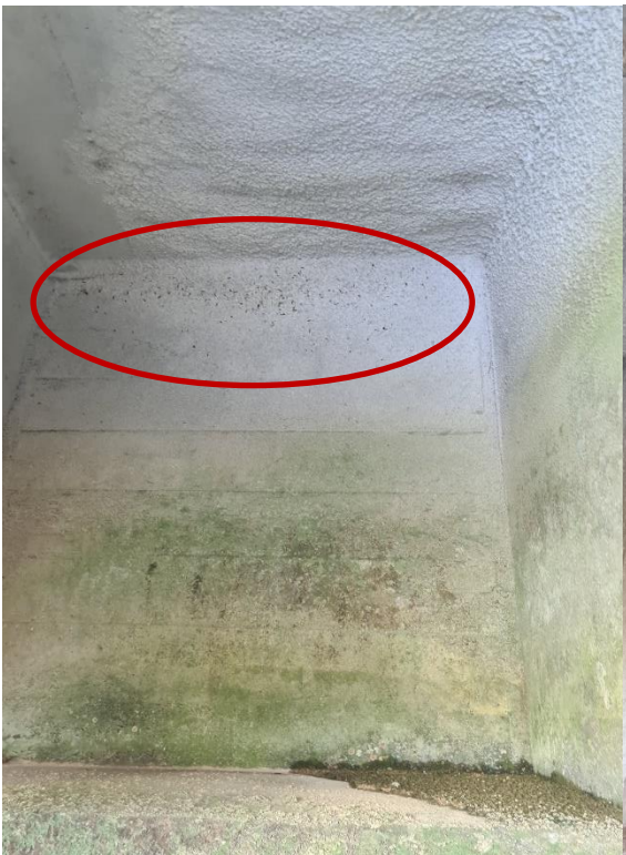
Plate 3-7: More bat droppings
