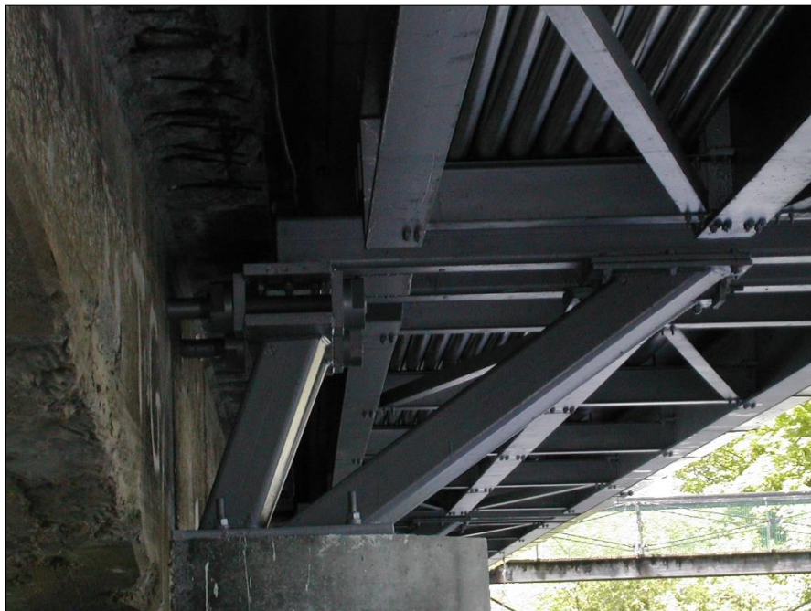
Photograph 2 - View of Existing Cantilevered Supports on the Upstream Side of the Bridge
