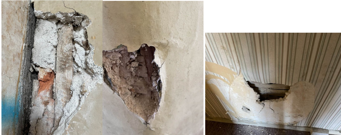
OBFA photos of existing internal wall finishes within the Manse (with varying substrates) and bulged finish
