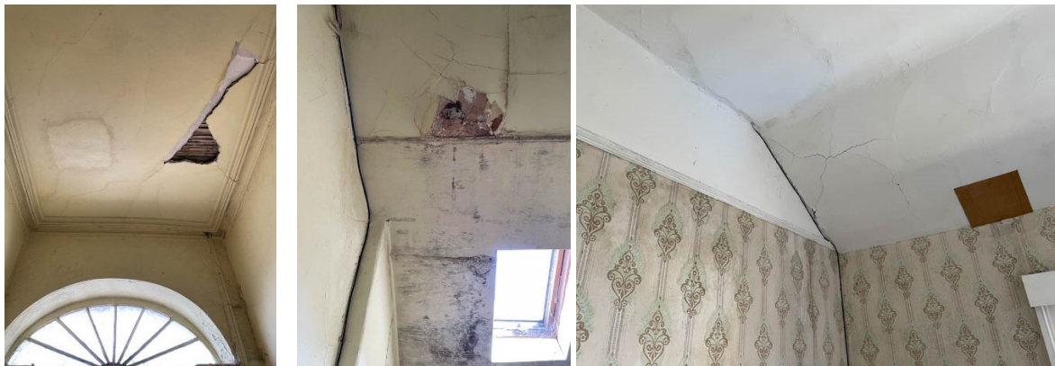
OBFA photos of existing internal ceiling finishes within the Manse -damaged areas / lath & plaster visible
