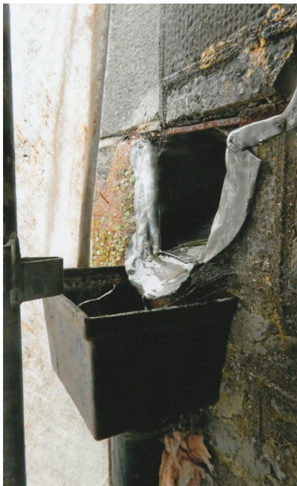
Fig. 7 The lead lined outlet from the parapet wall to the 1950's – 1960's hopper and downpipe. A larger diameter downpipe in cast iron will be required.
