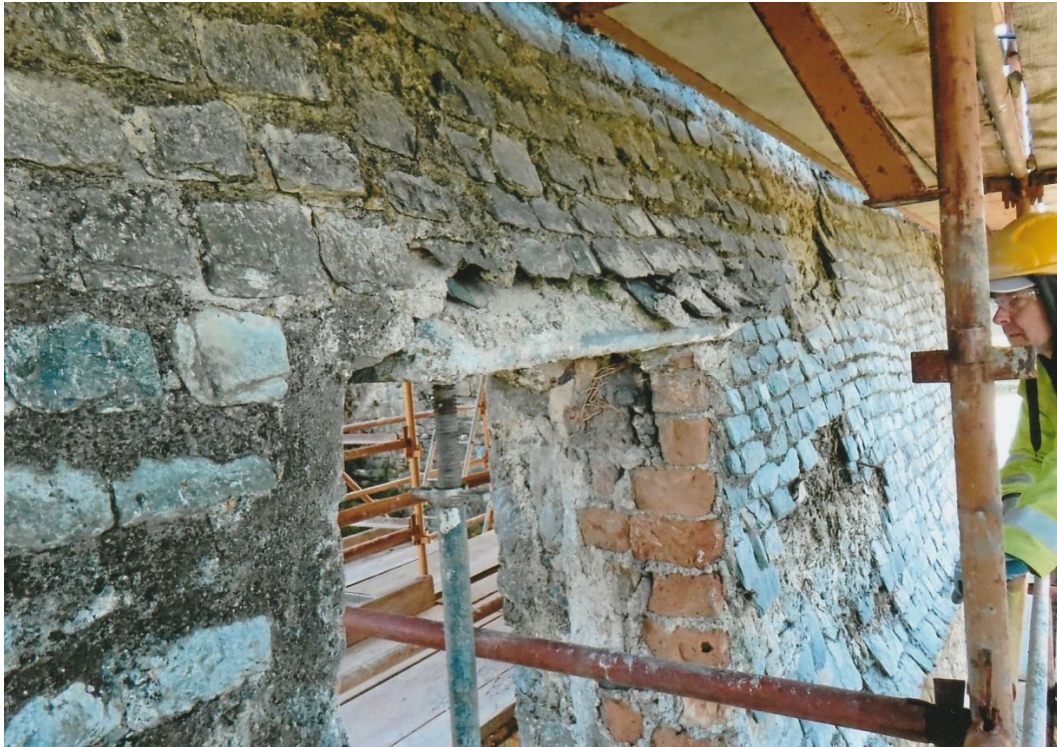
Fig. 78 Some of the inserted Georgian sash windows inserted on the River front of the 17 th and 18 th century block were precarious. An old limestone coping of some sort had been used as a lintel but did not fill the gap. The slate weather sheeting overlay it.
