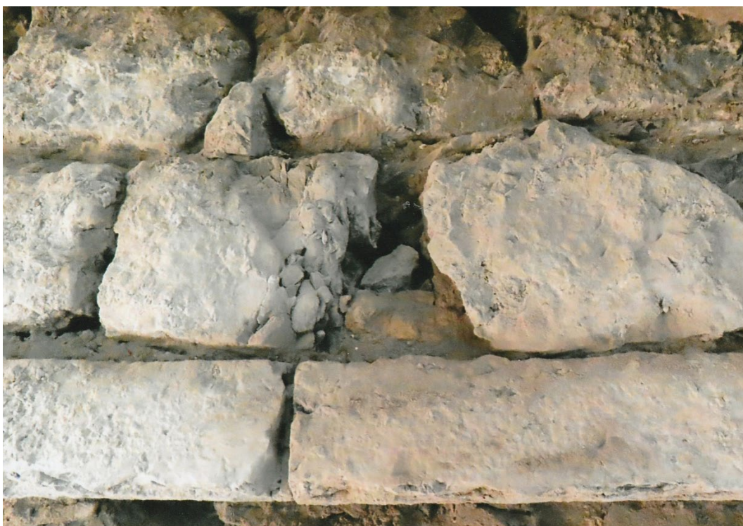
Fig. 57 A partially brick filled hole above the upper frame of the rectangular niche above the Flamboyant Lynch tomb. Photograph: J. Higgins.
