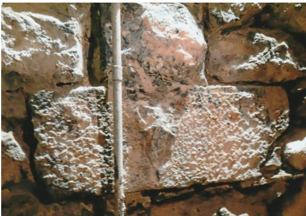
Fig. 33 The battered remnants of the left hand corbel / bracket which supported part of a gallery across the South end of the South Transept Extension. Photograph: J. Higgins.
