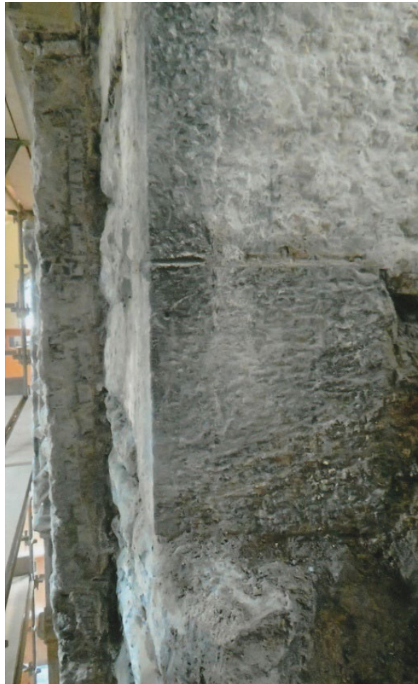
Fig. 43 The corner of the ingoing of the upper window on the east side of the east wall of the south Transept extension. The lower most stone on the left side has later tooling and may be a 19th century repair or insertion. Photograph: J. Higgins.
