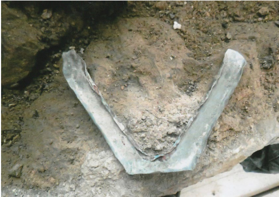
Fig. 50 A loose drip tray of copper alloy. These had been set in grooves cut with an angle grinder in the window mullions in the 1950's – 1960's works. Photograph: J. Higgins.
