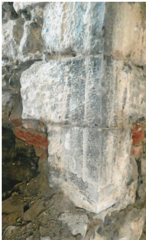
Fig. 45 Two lowermost stones on the right side of the upper window in the east wall of the South Transept Extension are retooled or 19th century insertions as is the red and yellow brick behind them. Note the binder of the lime-wash on the ingoing and outside it the line of the 1950's – 1960's render. A plain band was left outside of this on the sides of the ingoings and window soffits. Photograph: J. Higgins.
