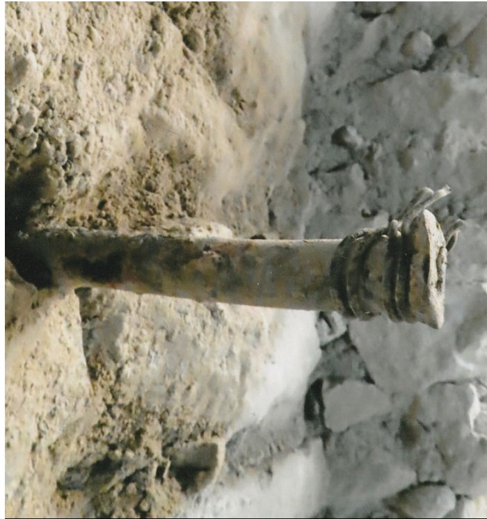
Fig. 58 Copper alloy spike, one of 14 metal pieces driven into the back wall of the niche over the Lynch tomb to help to hold the 1950's – 1960's shuttered concrete.
