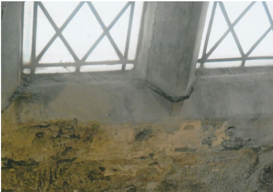
Fig. 51 The window mullions were smoothed with an angle grinder in the 1950's – 1960's and were cut with an angle grinder to insert copper alloy 'drip trays'. The intersection between the window and the mullions at the base, and the old glazing grooves were filled with cement. Photograph: J. Higgins.
