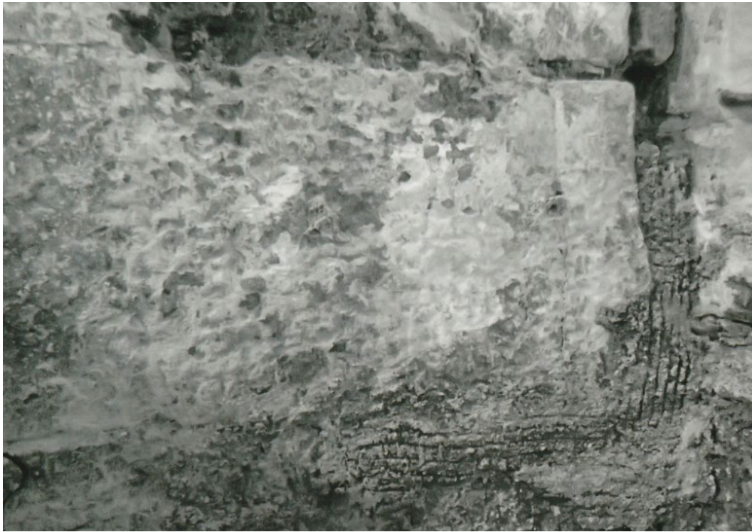
Fig. 44 Traces of lime-wash along with later small drilled holes and 1950's / 60's mortar filling in the ingoing of the lower window. The rough mortar filling was been striated to take the 1950's / 1960's cementitious mortar render. Photograph: J. Higgins.
