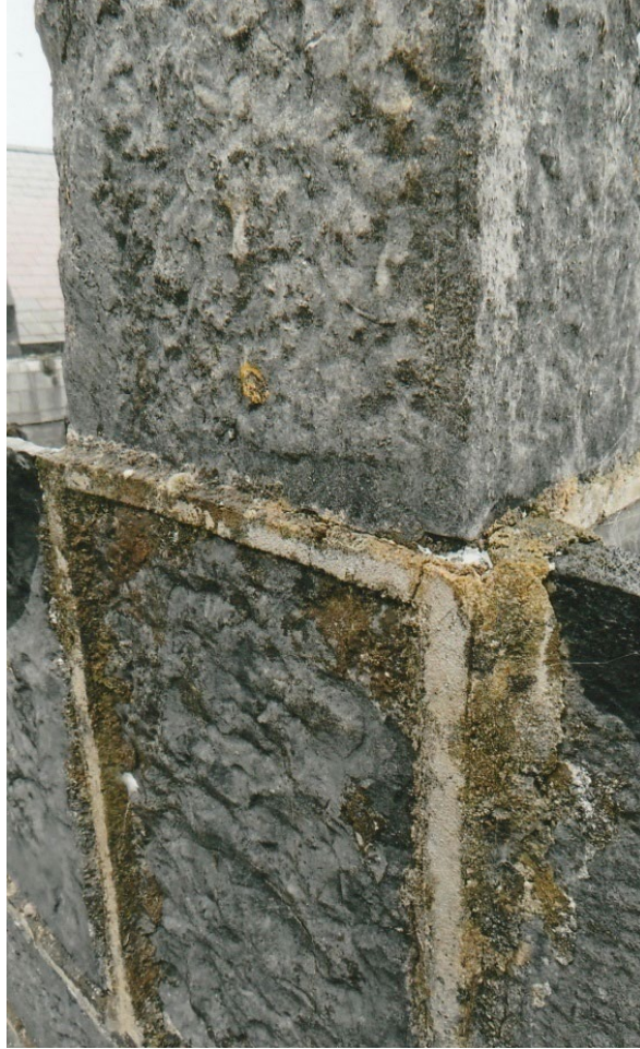
Fig. 9 Recent mortar raised strip-pointing was put over mastic in places. This has now been removed and replaced with a lime mortar mix set back in the joints. Photograph: J. Higgins.
