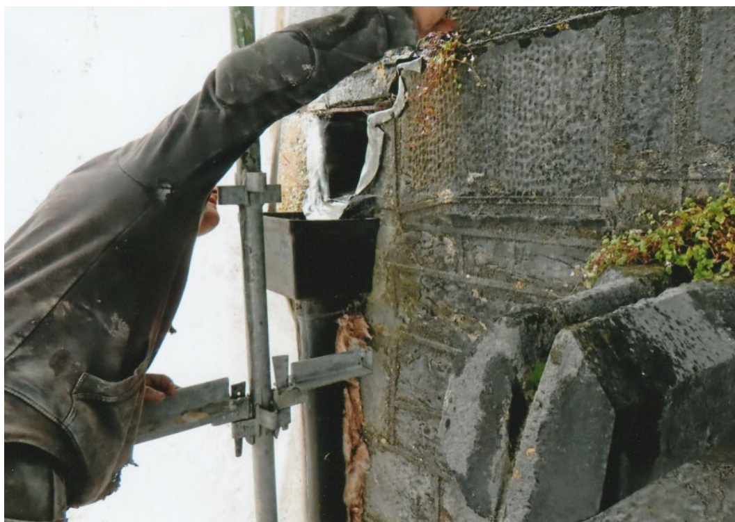
Fig. 6 The 19th century water spouts became defunct when a metal lined conduit was set behind the parapet and fed into the down pipes in the 1958-62 works. Photograph: J. Higgins.
