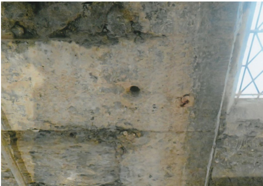
Fig. 52 A drill hole and a timber-filled drill hole with a nail at the side of the widow. Photograph: J. Higgins.
