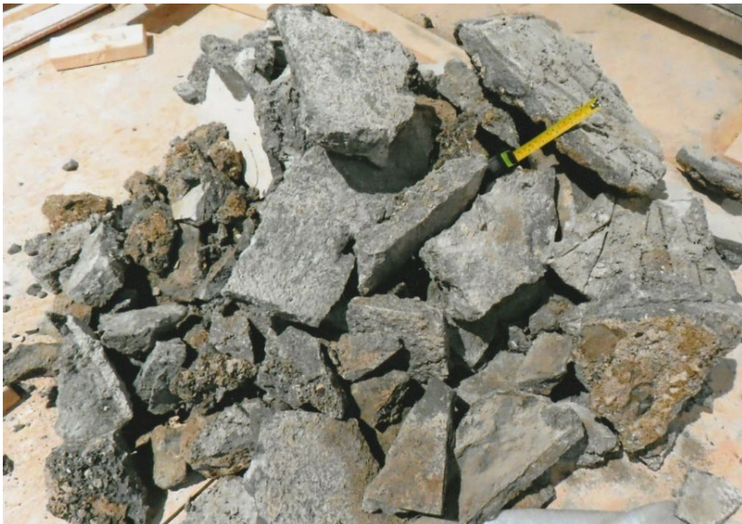
Fig. 12 Cementitious, mortar and stone along with degraded brown and grey mortar from the infill of the upper window of the South Transept Extension. Photograph: J. Higgins.
