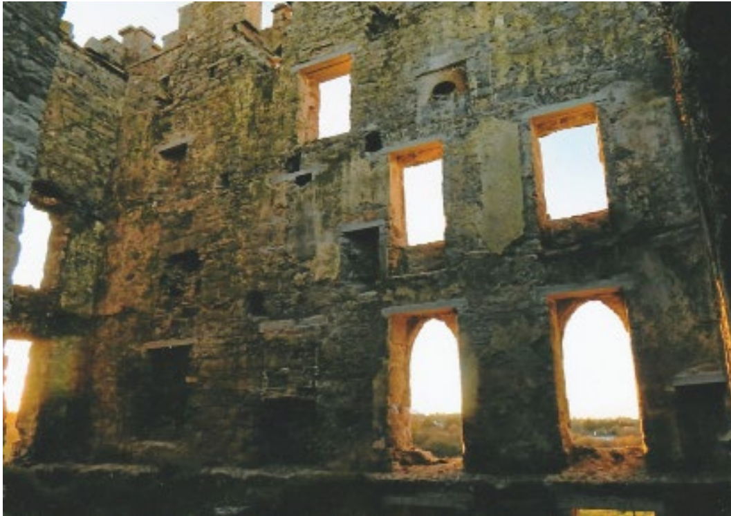
Fig. 93 Internal Work: Twelve of the rotted out and burnt wooden lintels visible in this photograph were replaced by limestone lintels in 2023. Photograph: J. Higgins.
