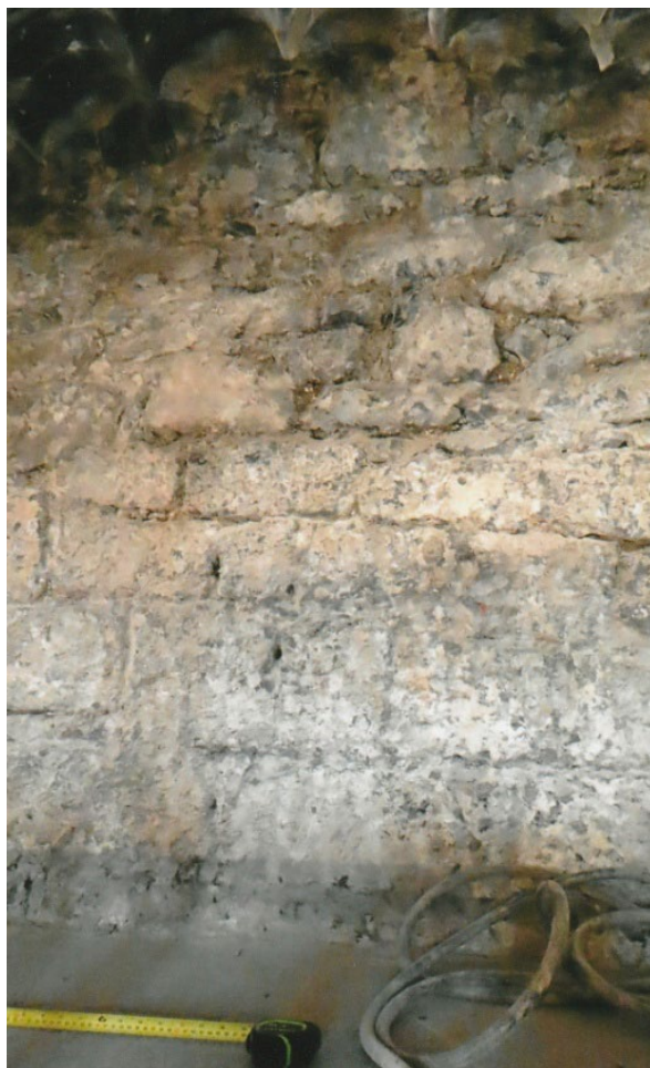
Fig. 5 Varied coursing and quality of stone used in the walling at the back of the flamboyant canopied and traceried Lynch Tomb seems to suggest two teams of masons or some rebuilding. Photograph: J. Higgins.
