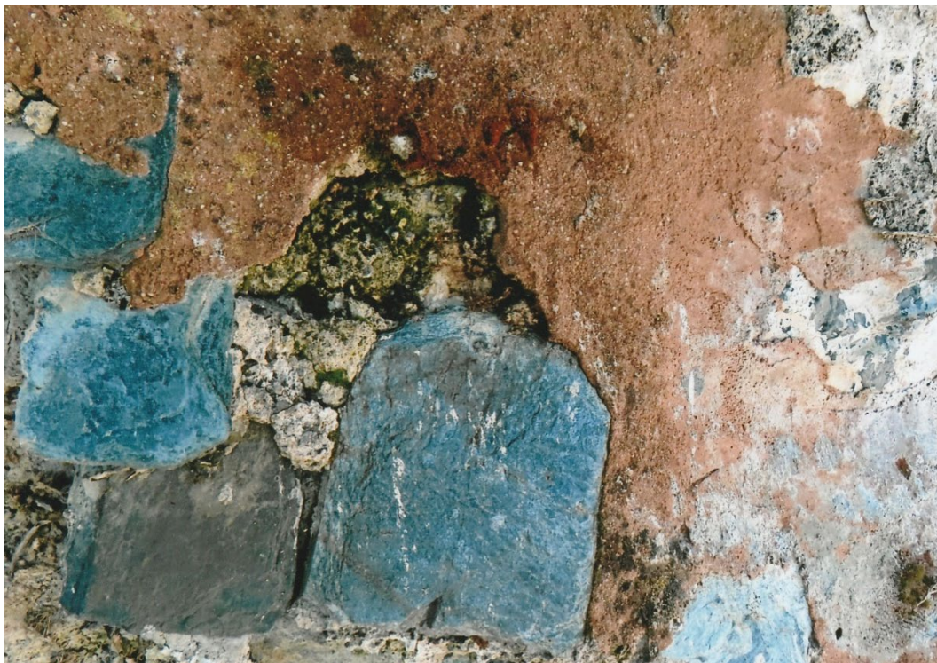
Fig. 83 Some areas of 19 th century repair with Roman Cement over earlier lime mortar and schist and grey slate weather sheeting at Menlo Castle.
