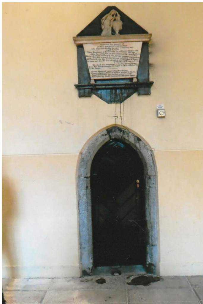
Fig. 70 Trapped moisture making its way from around a wall plaque and doorway onto the floor of the South Transept of St. Nicholas' Collegiate Church, October 2023. Photograph: J. Higgins.
