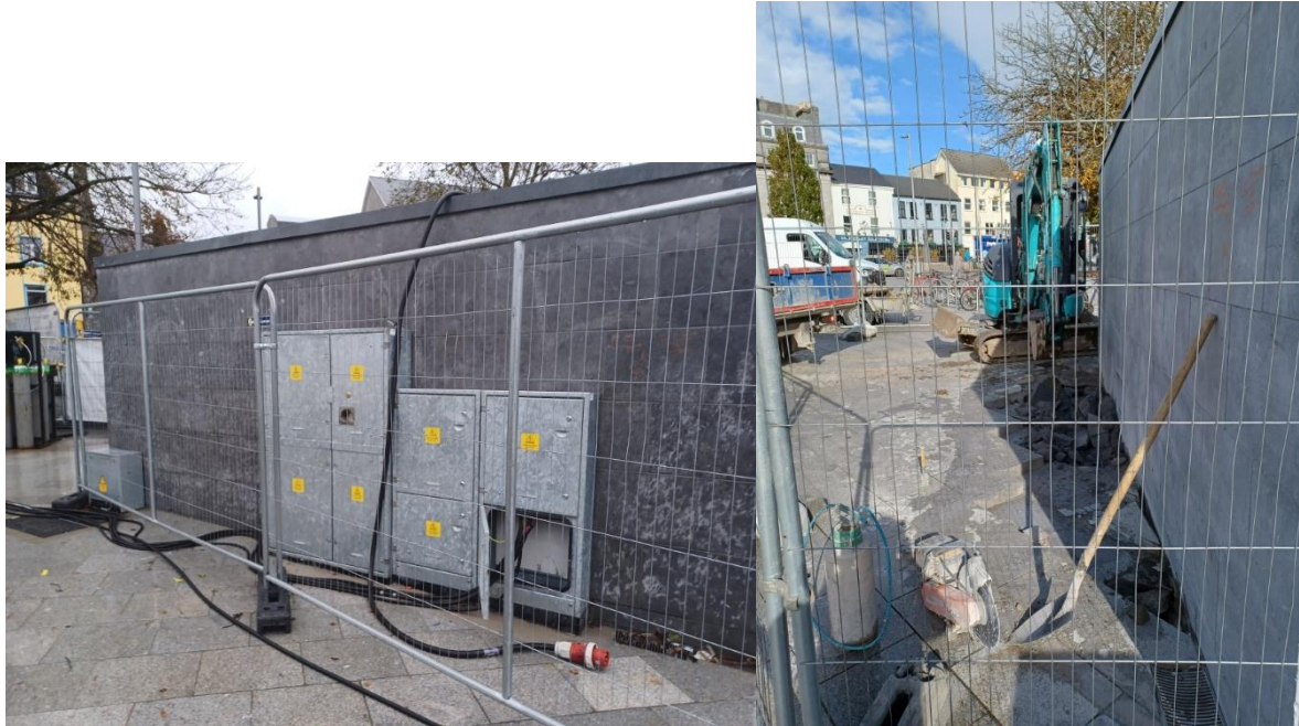
Photo of Eyre Square Sub-Station cabinet
